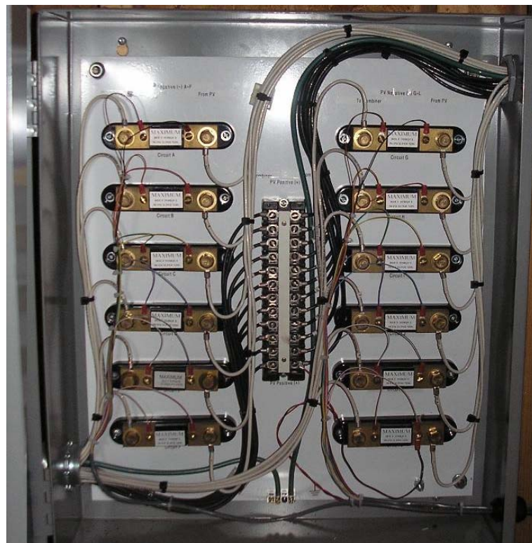
Figure 5. Current Monitoring Enclosure
