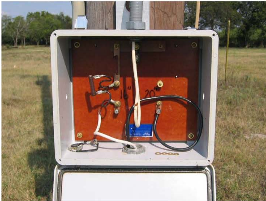
Figure 8. CP system disconnected at junction box
