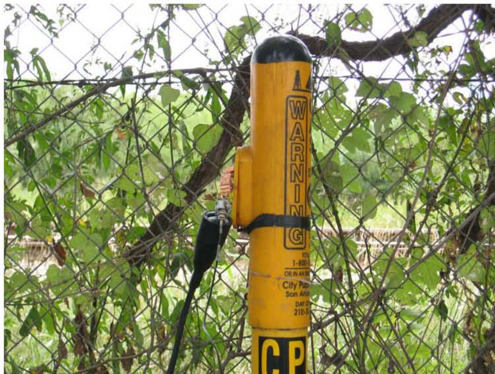
Figure 7. Connection clipped to test point on CP riser
