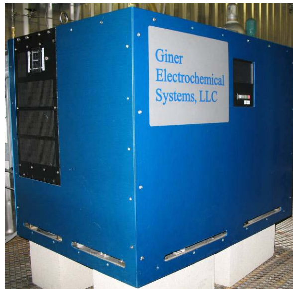
Figure 3 Giner's PEM-based Electrolyzer Module installed at NREL's Hydrogen Test Facility.
