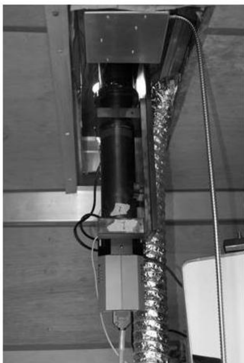
Figure 3.8: A SkyScanner (top) and MiniME FPI (bottom) are shown installed on the roof of a cargo trailer.
