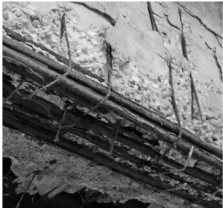
Figure 6. Beams deterioration on the side span
