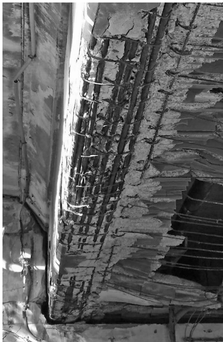
Figure 5. Beams deterioration on the side span
