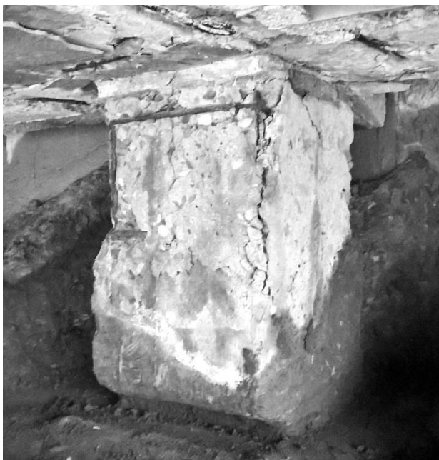
Figure 9. Deterioration and cracks on the concrete pendulum bearing
