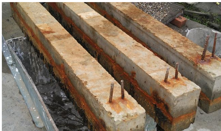
Fig 2. Stains on the beam surface due to corrosion
