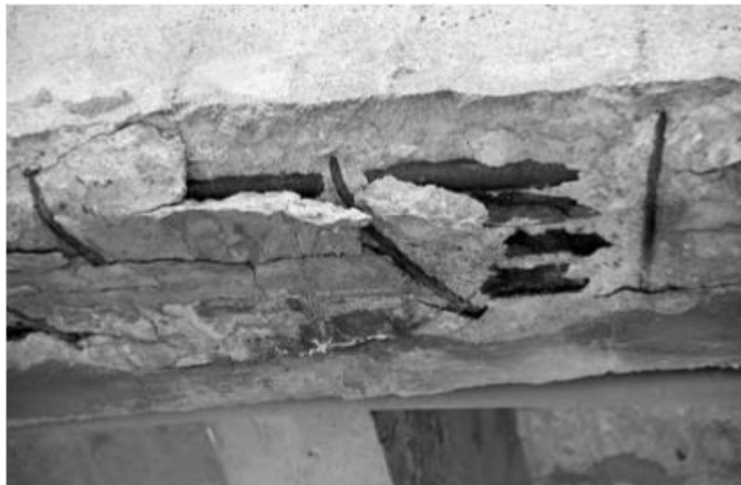
Fig 1. Corrosion of rebar in a RC beam
