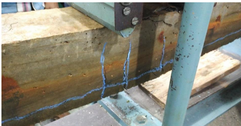
Fig 3. Cracking of concrete due to corrosion products (horizontal cracks)
