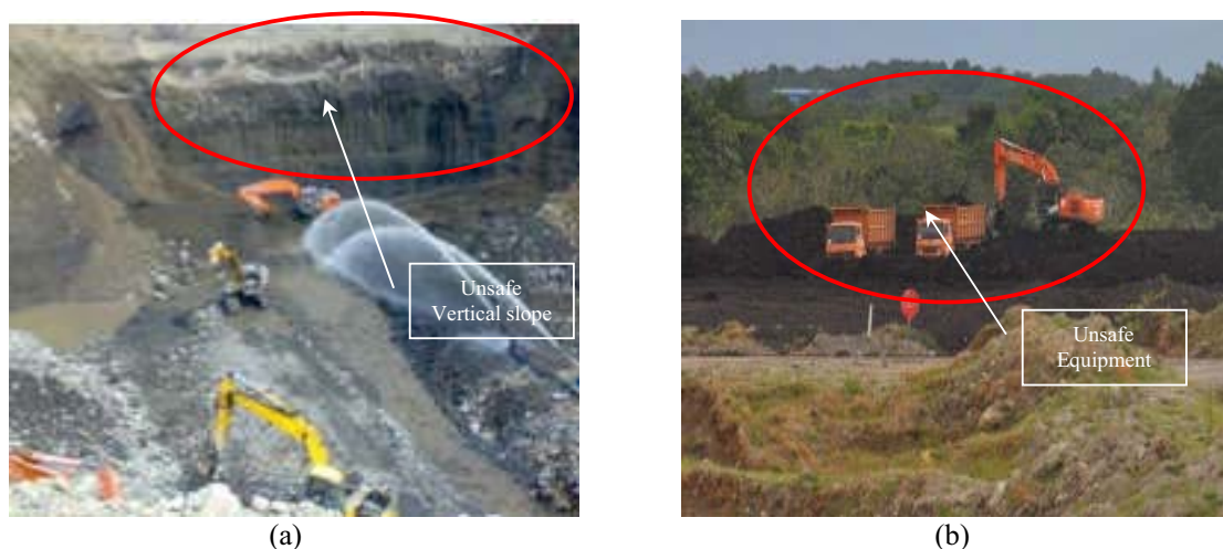
Figure 1. Unsafe Vertical slope (a) Critical Condition of the Coal Mining in Meureubo, (b) Unsafe Equipment (Bulldozer and truck) mobilization. The condition of coal harvesting place in Meurubo. [13]
