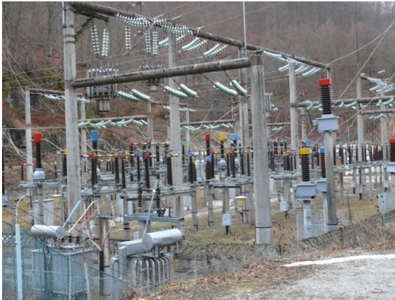
Figure 5. Devices and Bus Bars on H.T. level from Power Substation Remeti, Bihor
