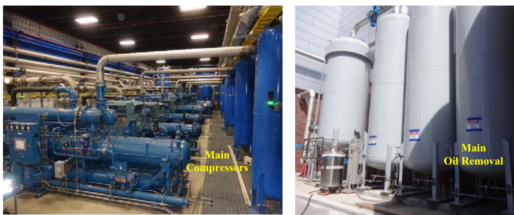
Figure 3. Main compressors and oil removal
