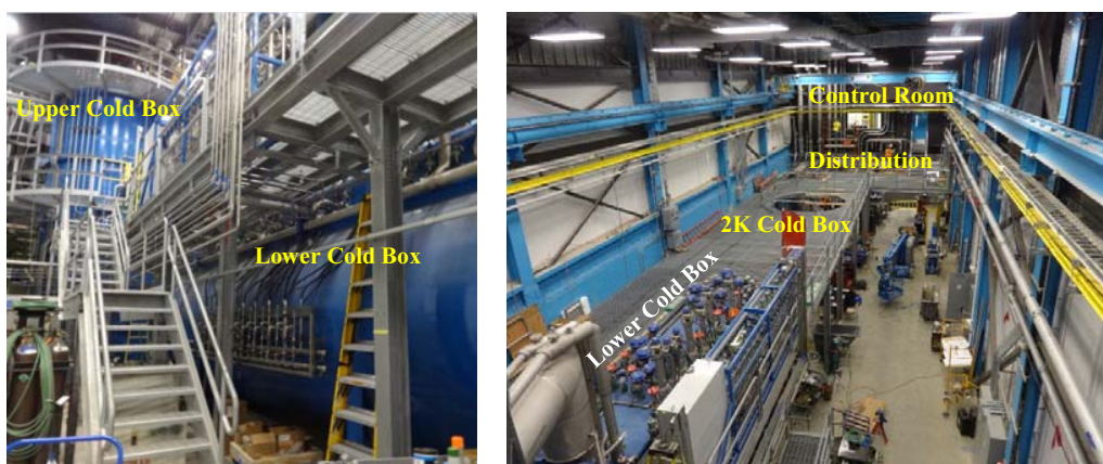
Figure 2. 4.5 K cold box and the cold box room
