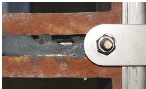
Figure 9. Incorrect filling of the mortar joint
