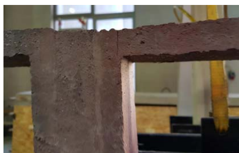
Figure 6. Cracking of clinker masonry unit as the result of the firing process during production
