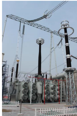
Figure 1. Transformer and casing above it (including corona ring)
