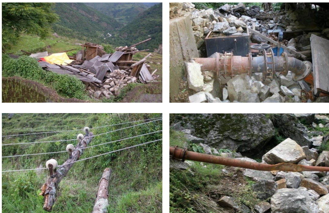
Figure 6. Micro-hydro plant damaged by the earthquake in Dolkha district in Nepal
