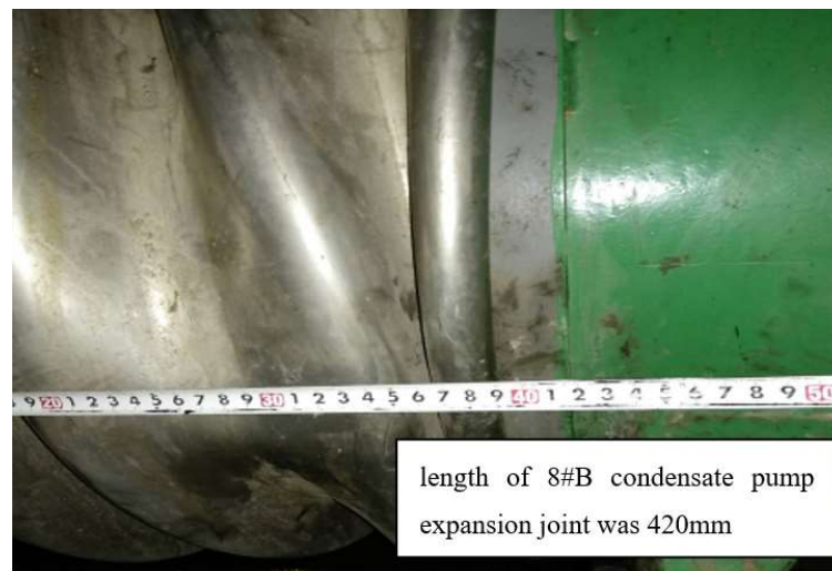
Figure 4. Deformation diagram of expansion joint at B condensate pump inlet.
