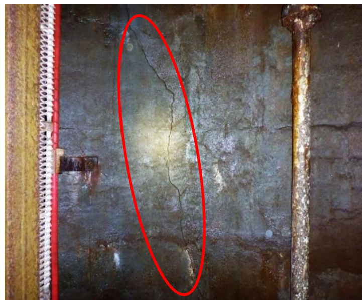
Figure 7. Example of vertical crack in concrete shaft liner.
