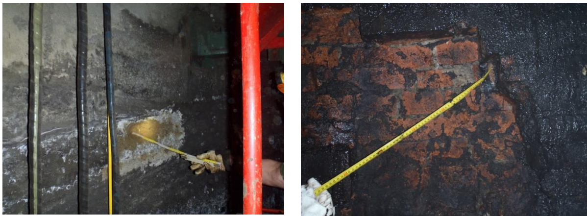
Figure 1. Cavities in concrete and brick shaft lining.
