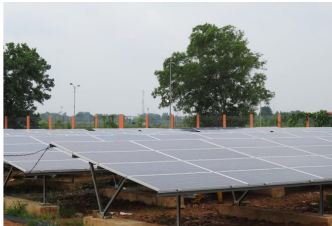
Figure 3. PV Power Plant in Palembang
