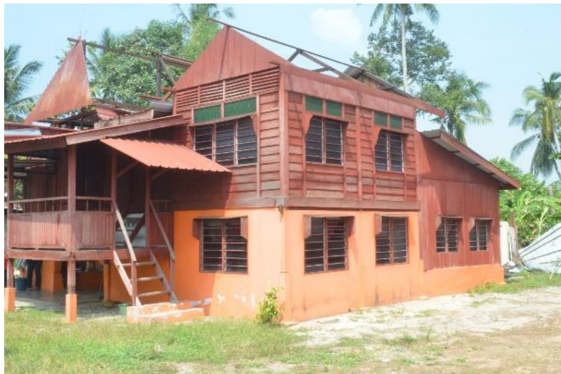
Figure 1. Example of roof uplift and damage timber trusses of a rural house in Penang, Malaysia
