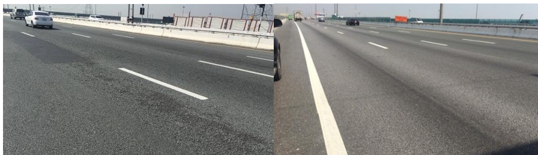
Plate 1. Ravelling & Pothole on PG76
