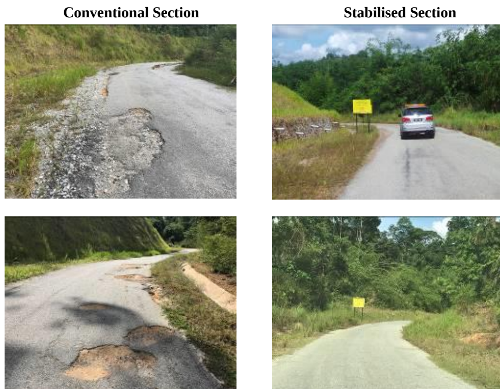
Figure 13. The condition at the site after 18 months.
