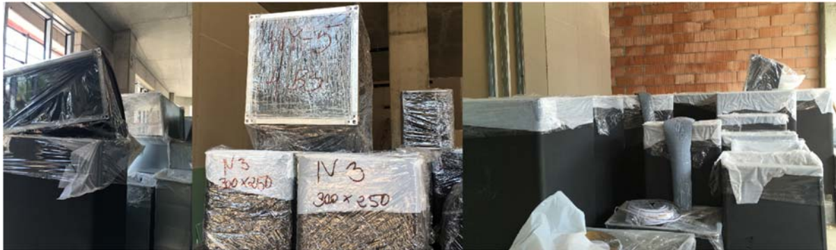
Figure 8. An example of the applied ventilation ducts at the storage stage [04.04.2017]
