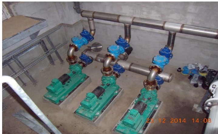
Figure 2. Influent pumps/wash filters
