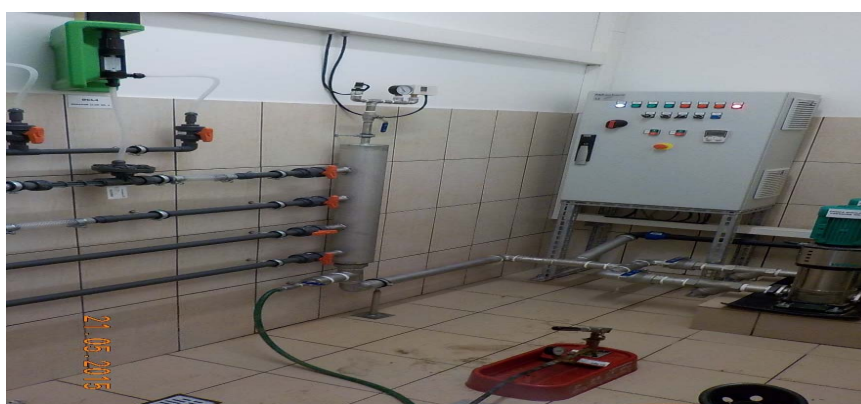
Figure 1. New chlorination station
