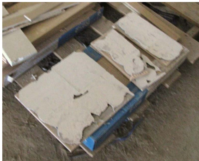
Figure 3. Tiles which came off with visible traces of gypsum on the layer of cement adhesive
