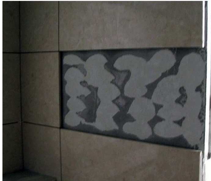
Figure 2. Wall surface after the tiles came off
