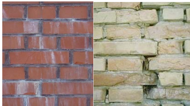
Figure 1. Exemplary effect of mortar corrosion
