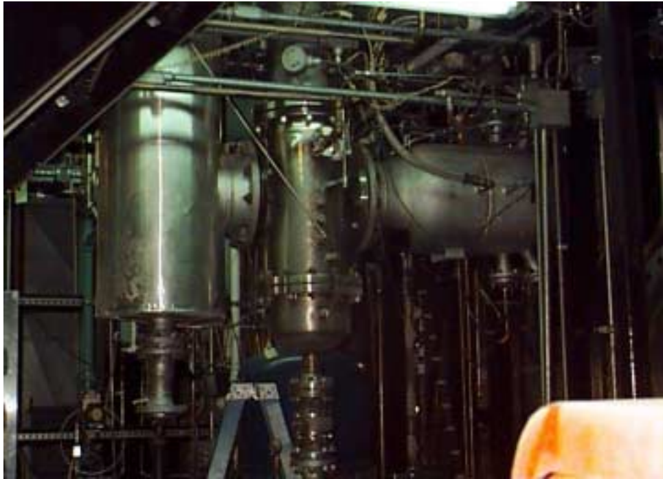
Figure 10. Filter Vessel Installed in Test Rig (center)
