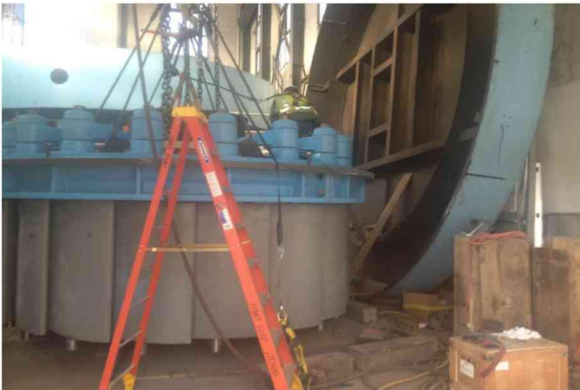
Figure 7. Refurbished Wicket Gate Assembly
